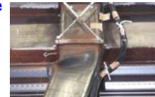
Local buckling at First Story Column Top
