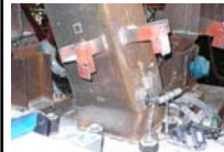
Local Buckling at Column Base
